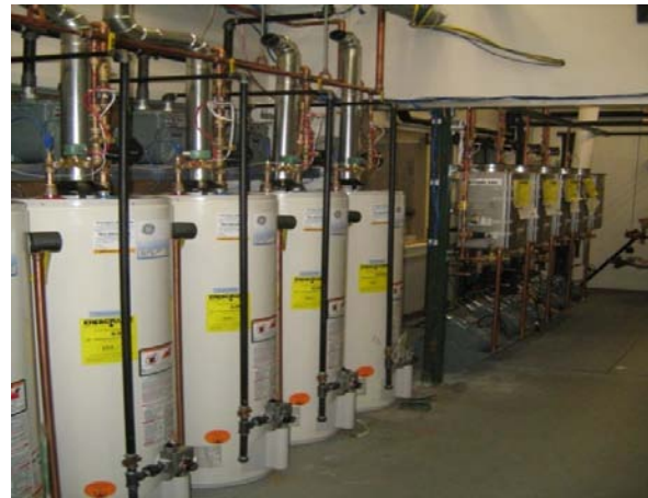
Figure 4-4. Gas Water Heaters
