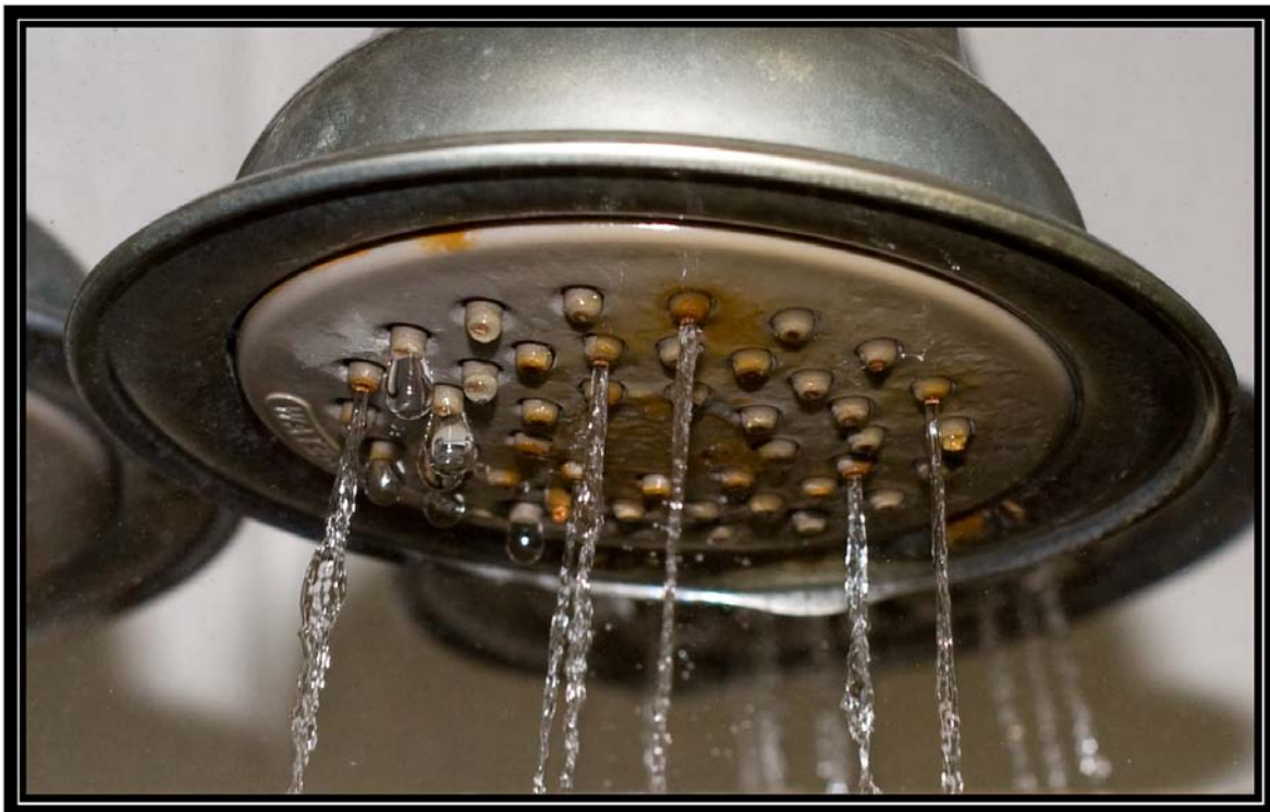
Figure 6-6D. Showerhead 6 on seventh day of testing with hard well water (28 grains per gallon) showing spray pattern. Battelle testing for Water Quality Association. May 1, 2009
